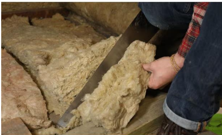
Insulation being laid in the attic of a house. An industry body says the levy on energy bills costs 52p a week, but saves an average of £300 a year for the 3 million homes who have benefitted. Photograph: Philip Toscano/PA
